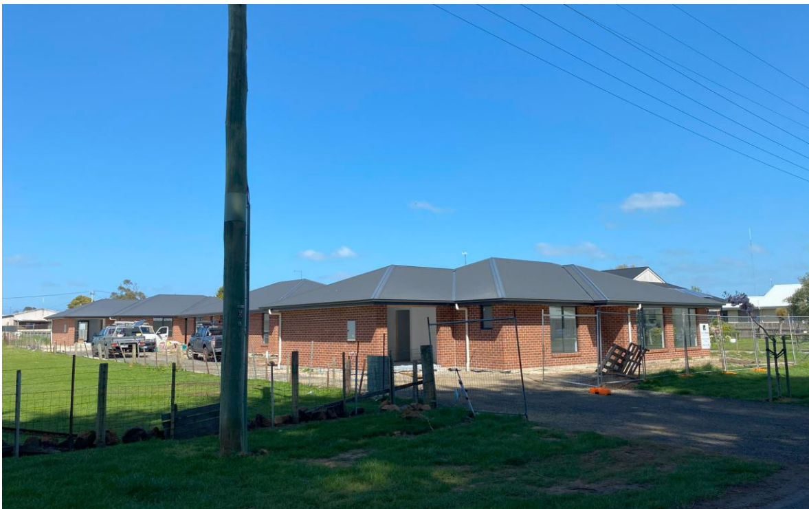
Figure 15: Multiple dwellings still in construction, no fence or landscaping or driveway (Source: David Cundall)
